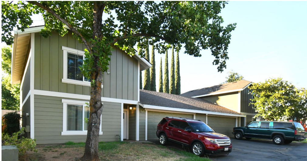
Evanswood Estates, Table Mountain Boulevard, Oroville - new façades. The $3 million exterior envelope work is substantially complete.
