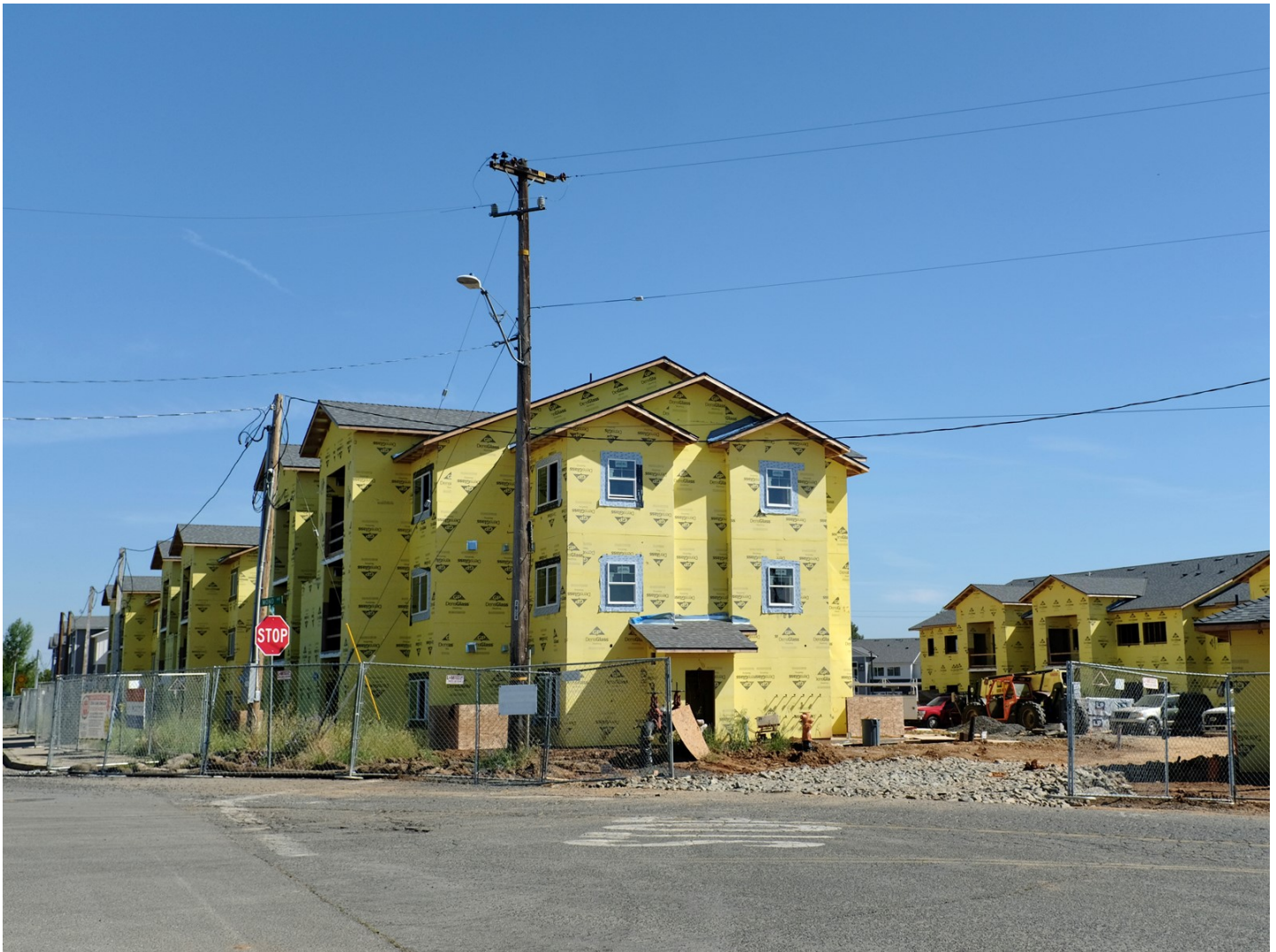
The Riverbend Family Apartments is seen under construction Wednesday on Table Mountain Boulevard in Oroville. MICHAEL WEBER — OROVILLE MERCURY-REGISTER
