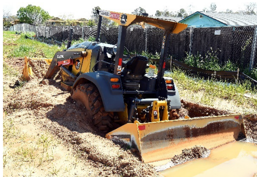
Prospect View Apts, Oroville – this is what rain does to building sites!
