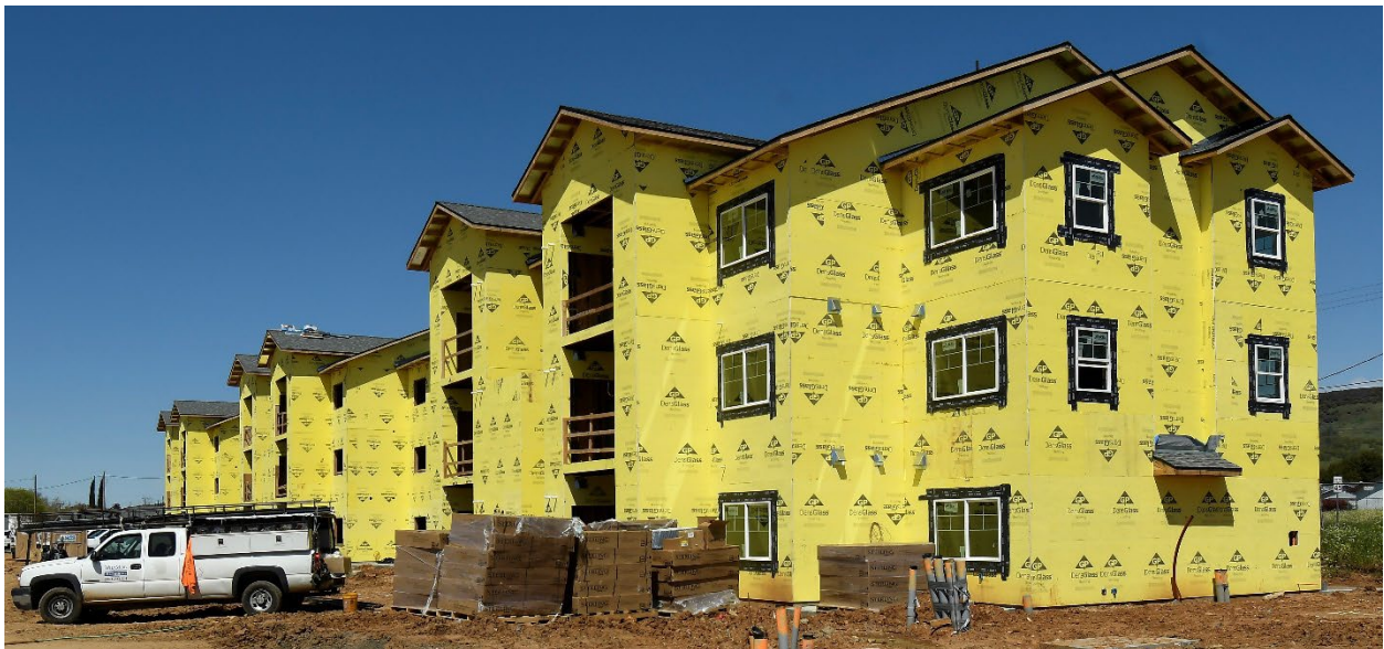
Riverbend II Apts, Oroville – framed up and roofed, waiting windows to complete building envelope
