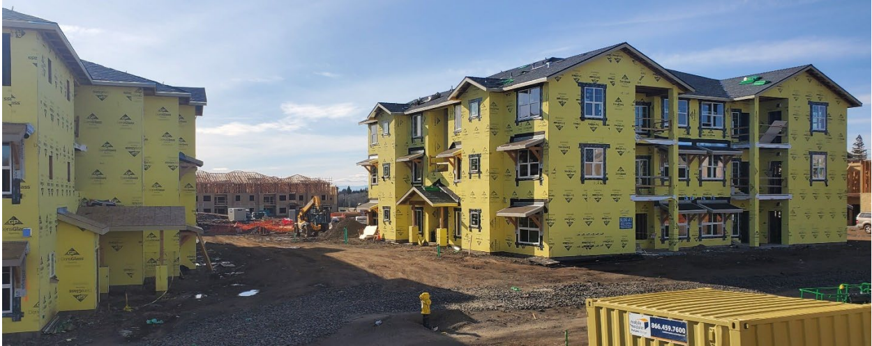
Deer Creek Apts, I, Chico – framed, roofed, and closed in. Ready for interior and exterior finishes.
